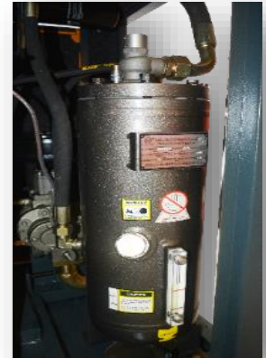
Oil separation Chamber
