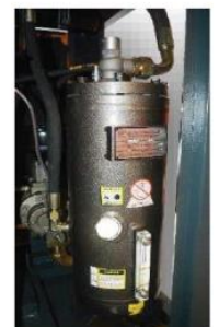
Oil Separation Chamber
